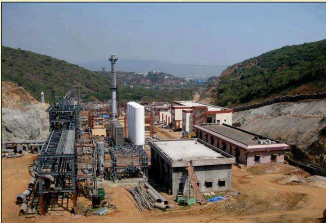
View of the aboveground facilities at Visakhapatnam
